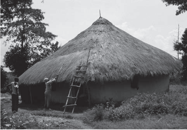
Figure 15. Man performing roof repair on his wife's house. Only men are allowed to climb onto the roof.
